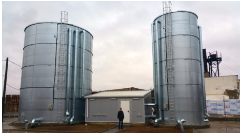
An Eco Avangard SRL Water Treatment Plant
